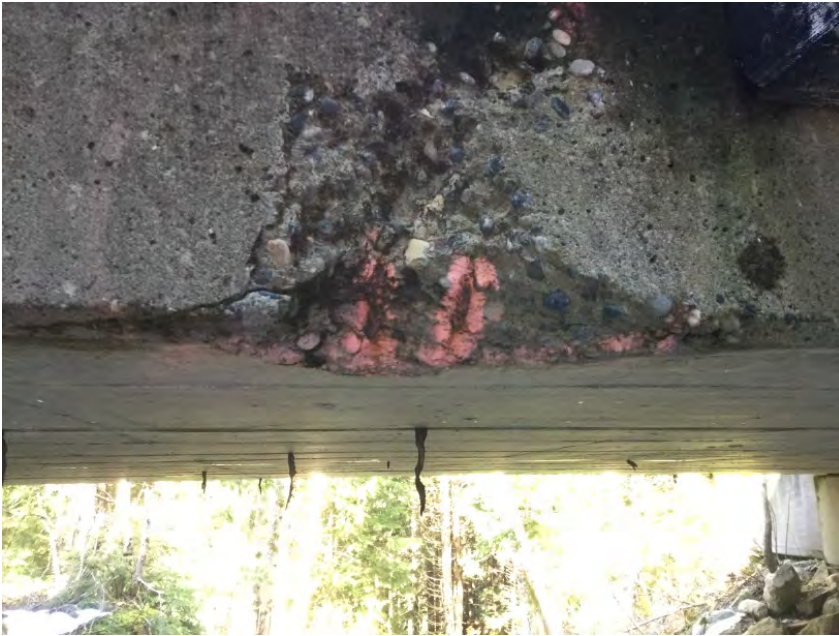
Damage to upstream concrete slab
